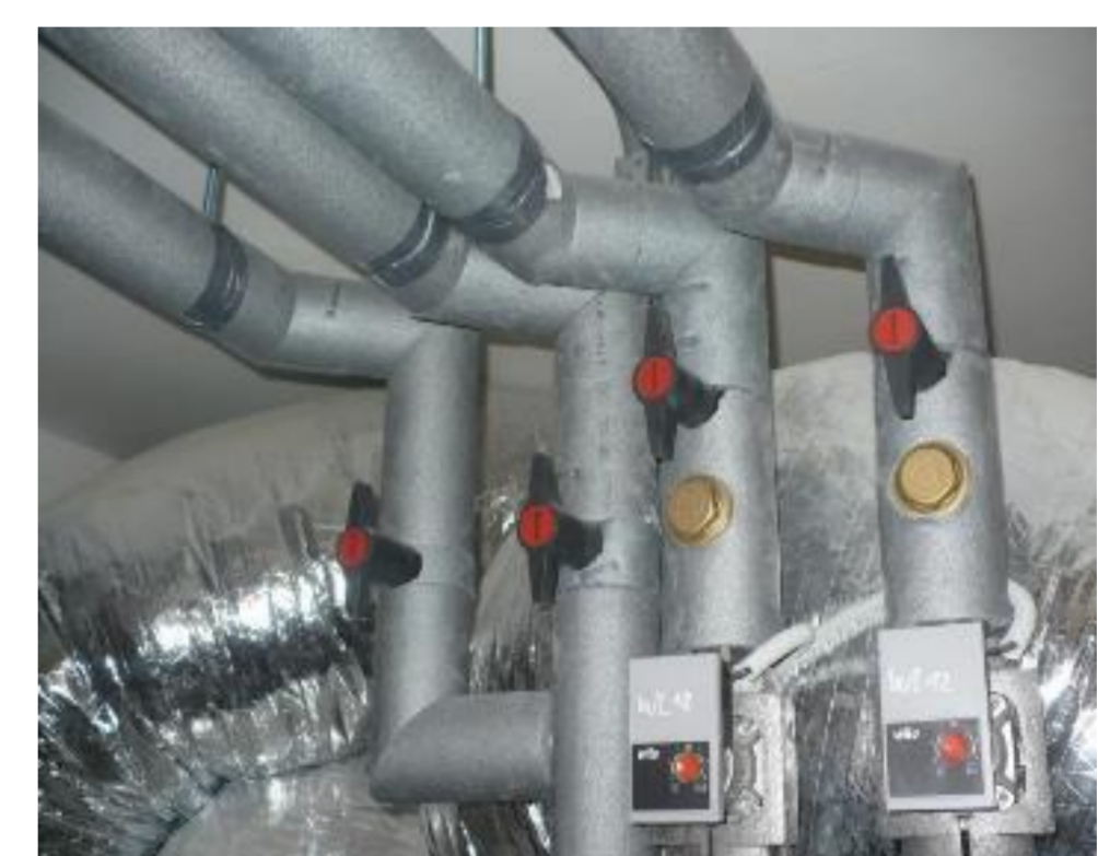
PV supported air-to-water heat pumps in Bratislava
